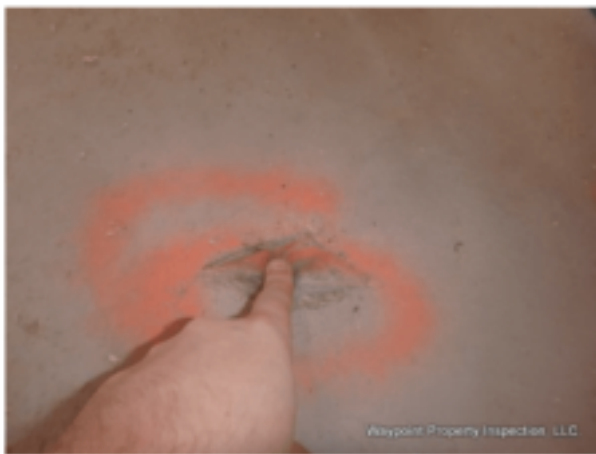
Exposed vapor barrier was present at kitchen in less than 1/4 inch of concrete.
