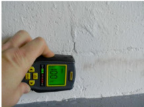
Moisture stains were visible. The stains tested wet using moisture meter.
