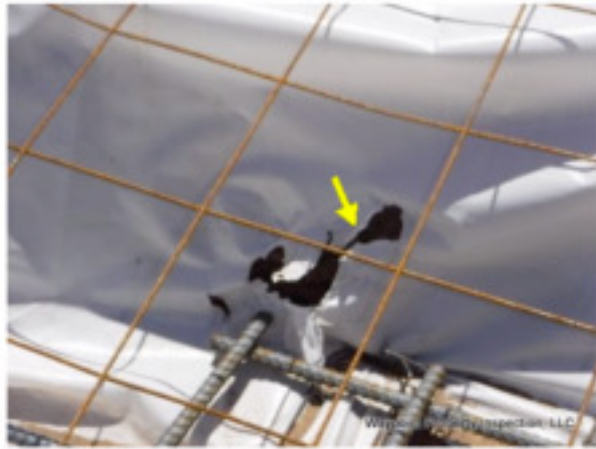
Minor holes were visible in visqueen vapor barrier.
