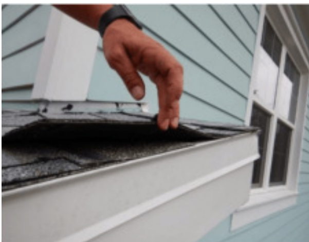
Loose shingles/covering were visible.
