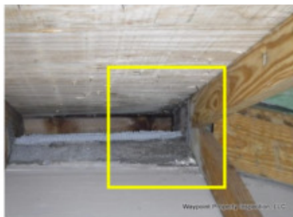
Moisture stain(s) were visible at the accessible areas of the garage attic. Stain was visible at garage ceiling.
