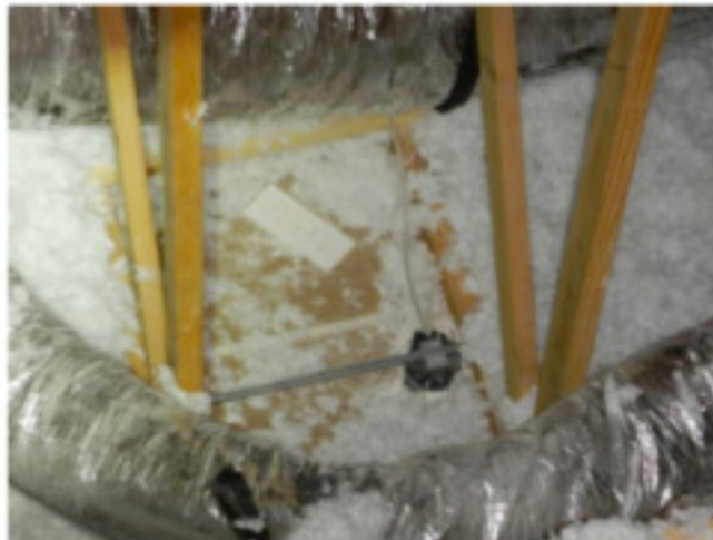
Insulation had been moved/disturbed, leaving low coverage areas.
