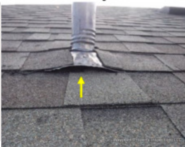
Loose roof covering was visible.
