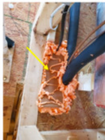
Cardboard was being used as a fire block.
