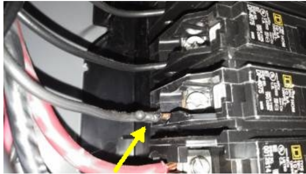
Damaged wiring was visible.
