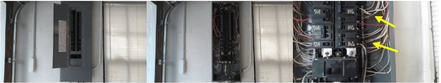
Two wires (double tap) connection was visible.
