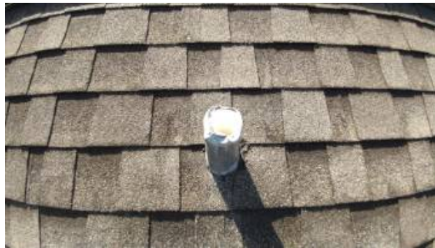
Vent cap(s) were damaged.
