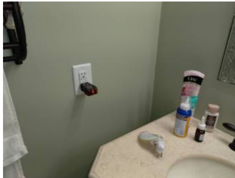
GFCI (Ground Fault Circuit Interrupter) outlet(s) was damaged at master bathroom.
