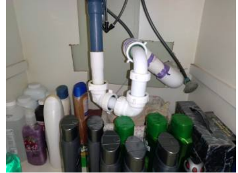
Traps were improper/not present at master bathroom.
