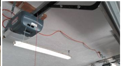
Extension cord was improperly used as hard/permanent wiring at garage.
