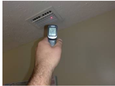
Supply air temperature
