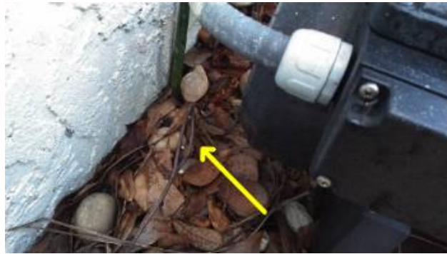
Body bond was loose/improperly secured at the pump.
