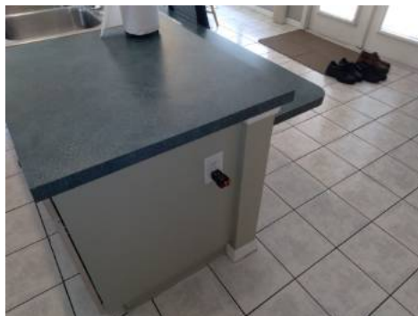
GFCI (Ground Fault Circuit Interrupter) outlet(s) should be installed at en suite kitchen island outlet.
