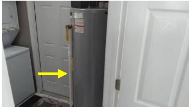
Temperature pressure relief valve (TPR Valve) piping was improper. (CPVC Required)
