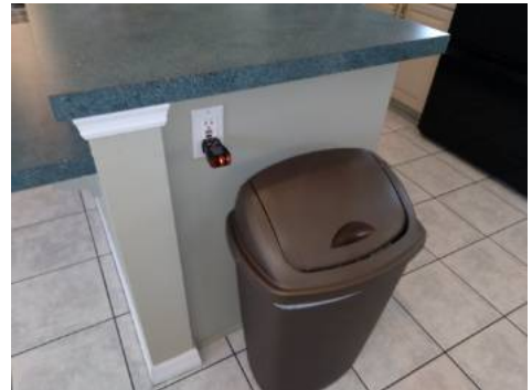
GFCI (Ground Fault Circuit Interrupter) outlet(s) was damaged at en suite kitchen island.
