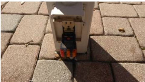
Outlet(s) were not operational at the porch.
