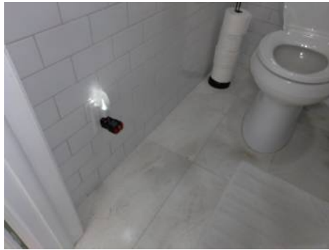
Outlet(s) tested not properly grounded at master bathroom.
