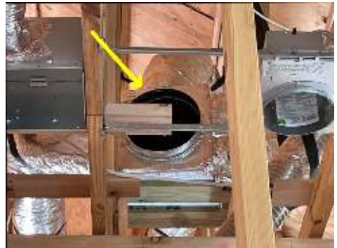
Ducts were not installed at various areas.
