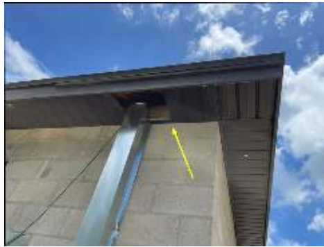
The soffits were damaged.
