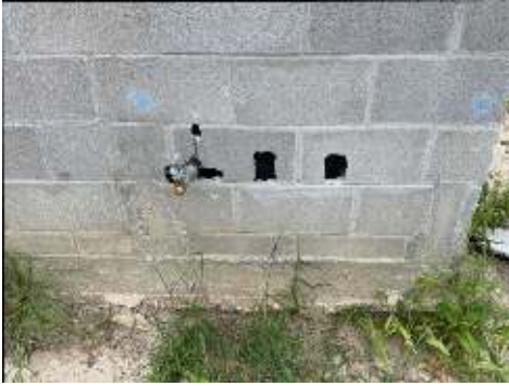
Holes were visible.
