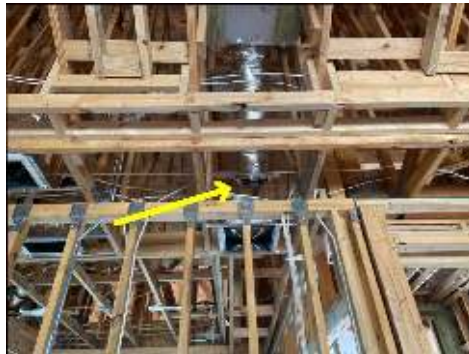
Ducts were not installed at various areas.
