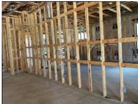
GFCI outlets rough wiring appeared serviceable.
