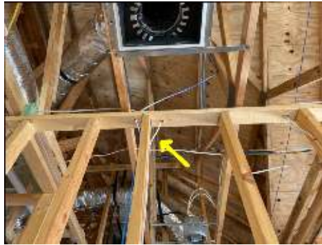
Fire block was not installed at the time of inspection
