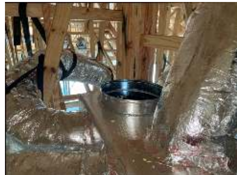
Ducts were not installed at various areas.
