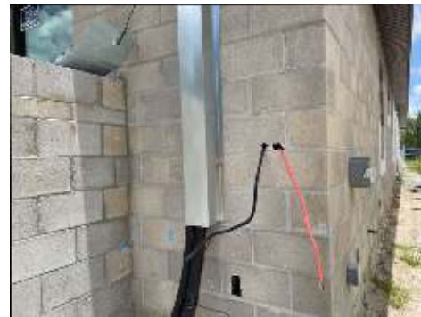
Electrical disconnect rough wiring appeared serviceable.
