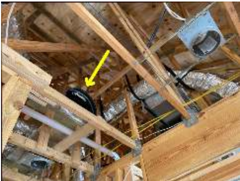
Ducts were not installed at various areas.
