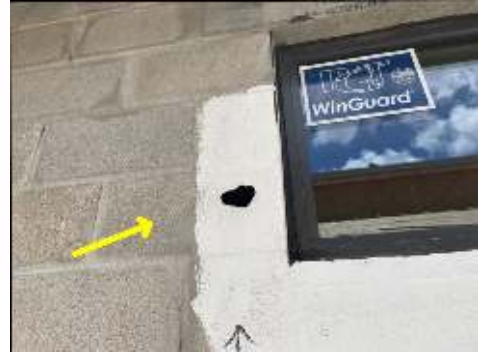
Holes were visible.
