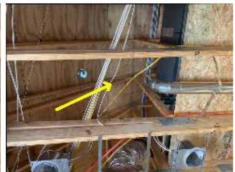
Dryer vent was not properly secured/sealed.
