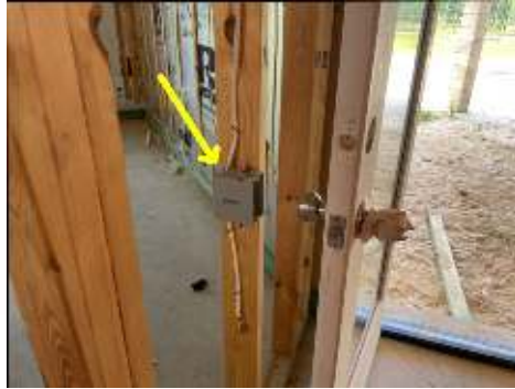
Outlet is in danger of being damaged.
