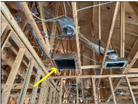
Ducts were not installed at various areas.
