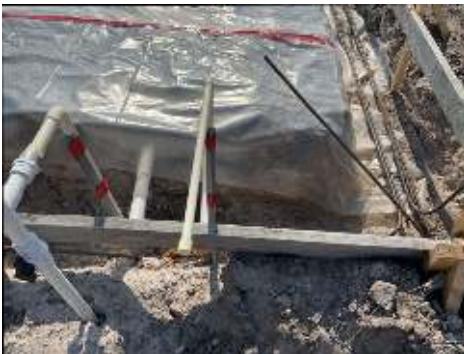
Exterior Faucet supply piping
