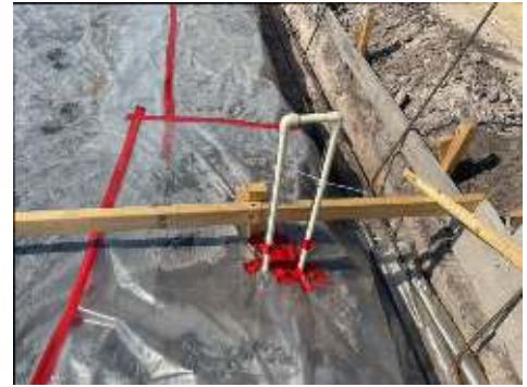
Water Heater supply piping
