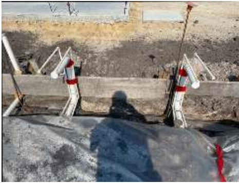
Master Bathroom supply piping
