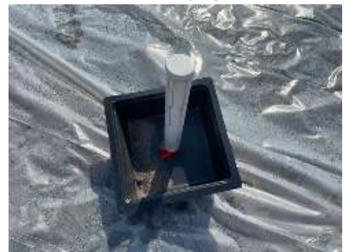
Master Bathroom drain piping
