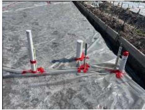
Secondary bathroom supply piping
