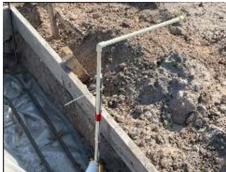
Exterior Faucet supply piping
