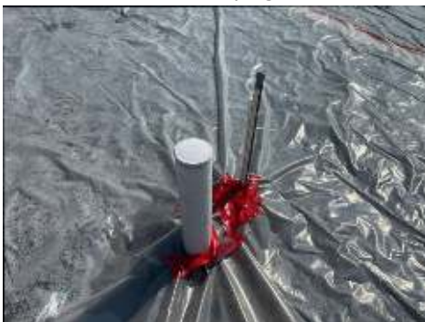
Master Bathroom drain piping
