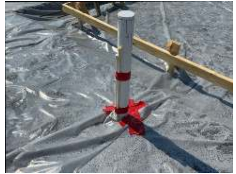
Laundry drain piping
