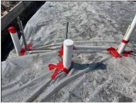
Secondary bathroom drain piping
