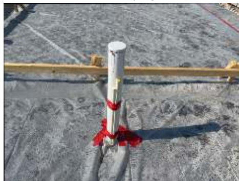
Master Bathroom drain piping
